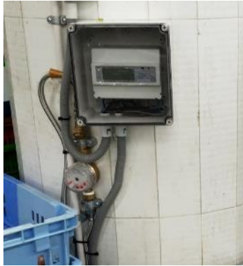
Electric & Water Meter
