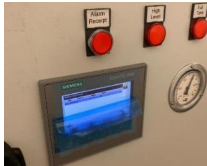
System Control Panel
